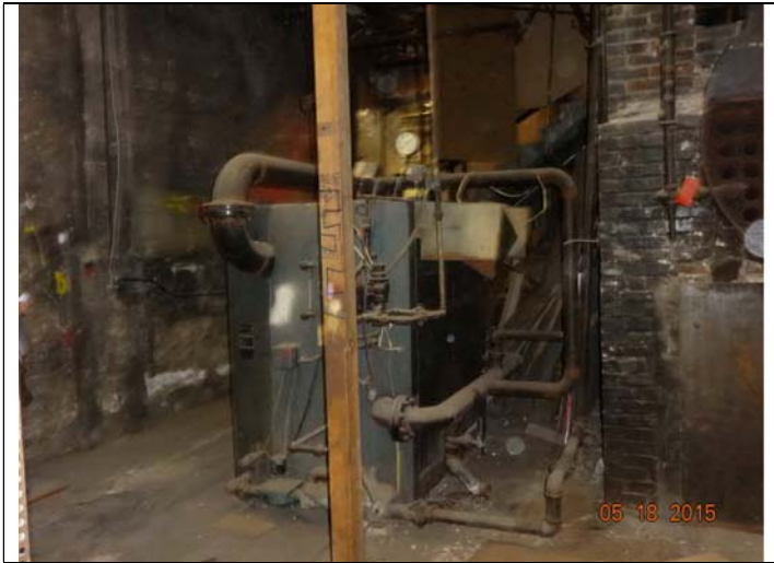
25. View of boiler.
