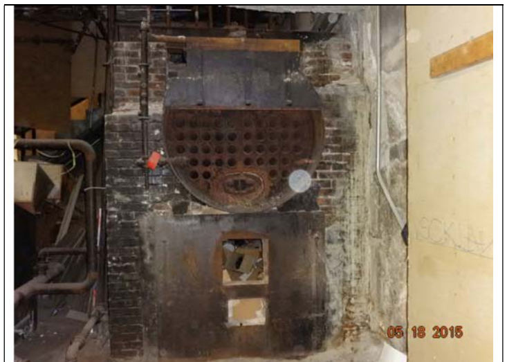
24. View of furnace
